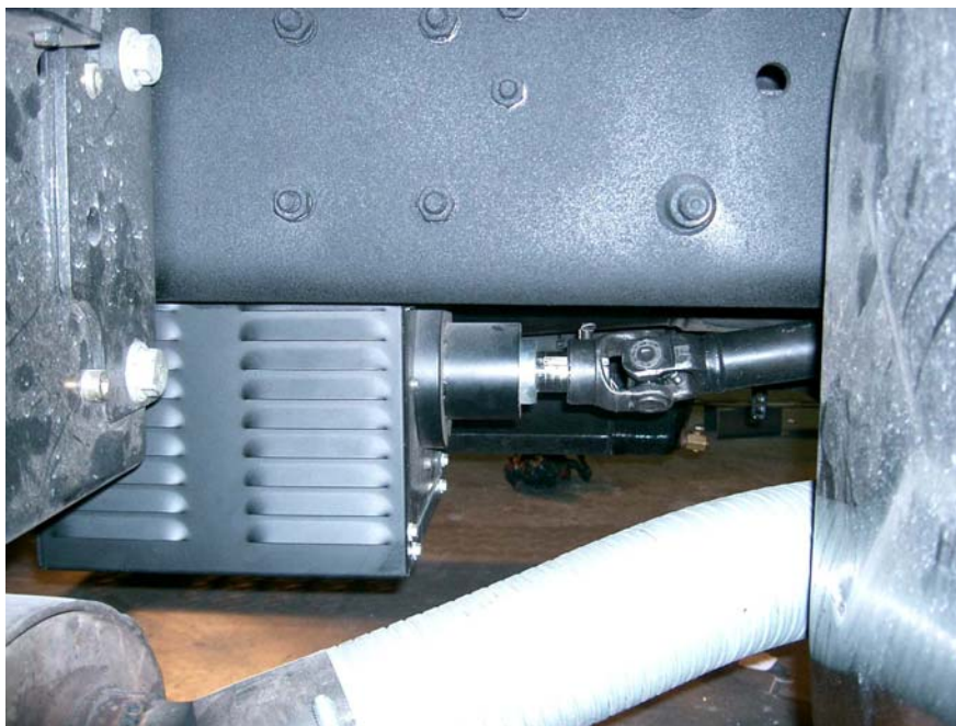
Figure 5-7: PTO Auragen Generator
