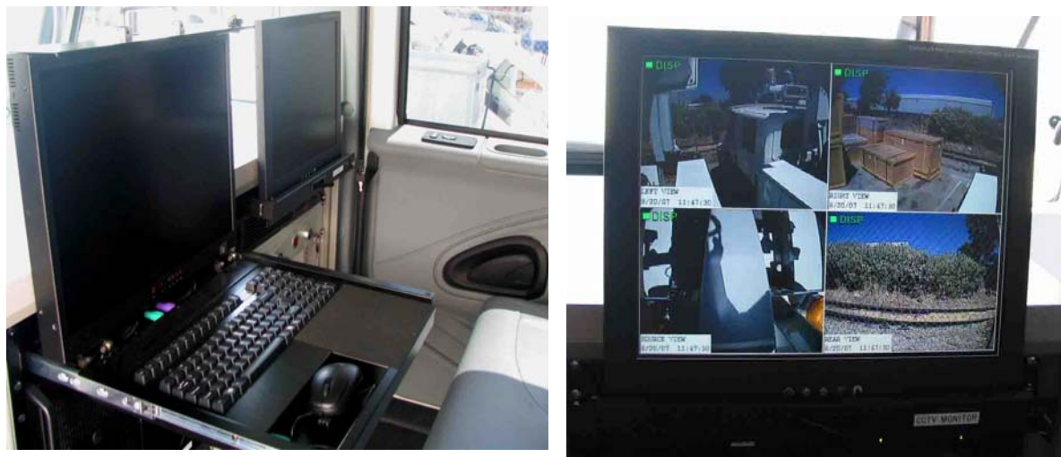
Figure 3-7: Closed Circuit TV System and CCTV Camera views
