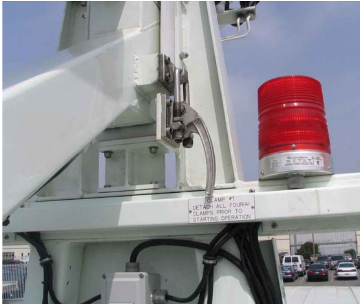
Figure 12-5: Clamp #1 above the light bar
