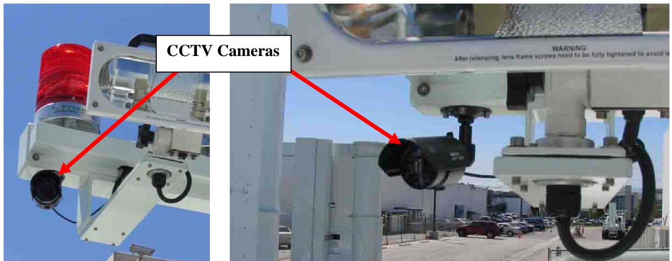
Figure 3-5: CCTV Cameras on Light Bar
