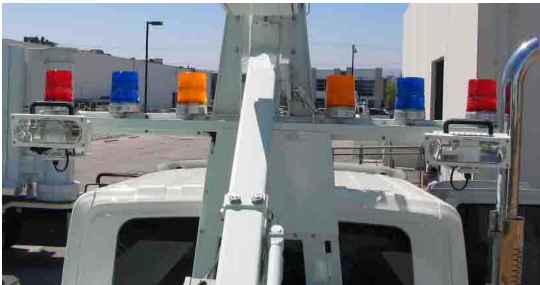
Figure 3-9: Gamma ray Source Warning Lights
