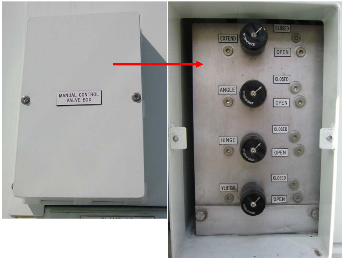
Figure 12-12: Manual Control Valve Box
