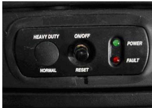
Figure 5-8: Generator Power Switch
