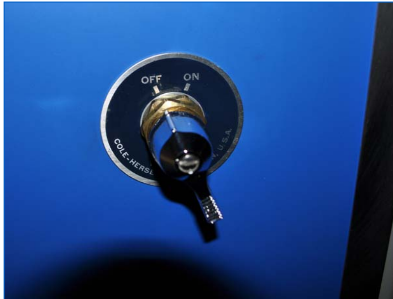
Figure 38: Master Battery Disconnect
