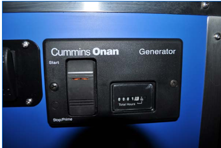
Figure 78: Remote Generator Start-up
