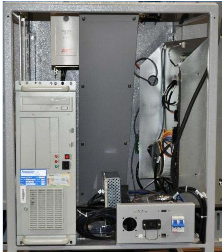
Figure 44: Electronics Cabinet and main circuit breaker
