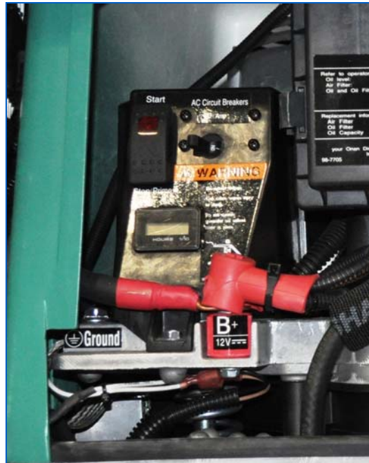
Figure 20: Local Generator Controls
