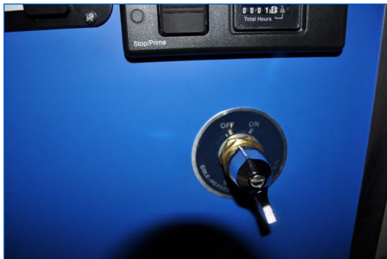
Figure 79: Master Battery Disconnect
