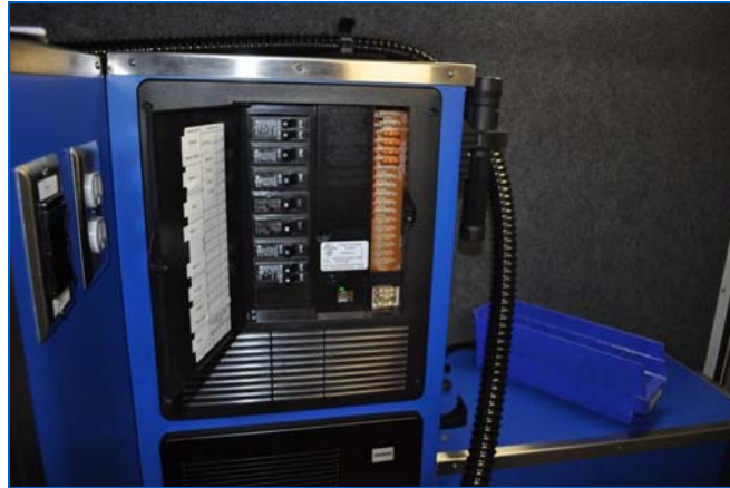
Figure 72: Circuit Breakers in the Off Position
