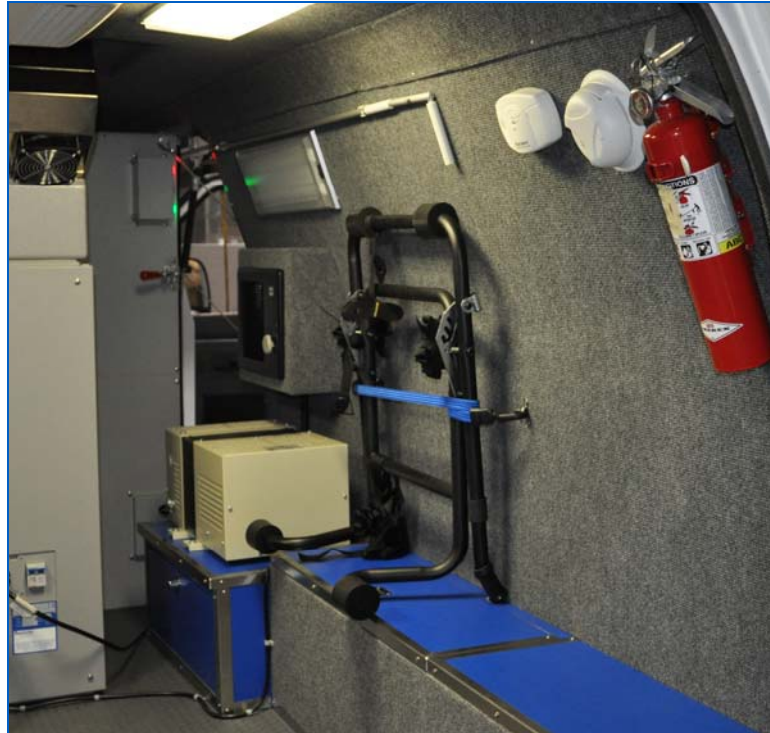
Figure 51: Operator Station Support Rack
