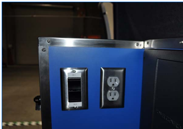
Figure 39: Heater Control and Electrical Outlet
