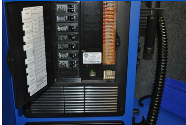
Figure 73: Circuit Breakers in the On Position
