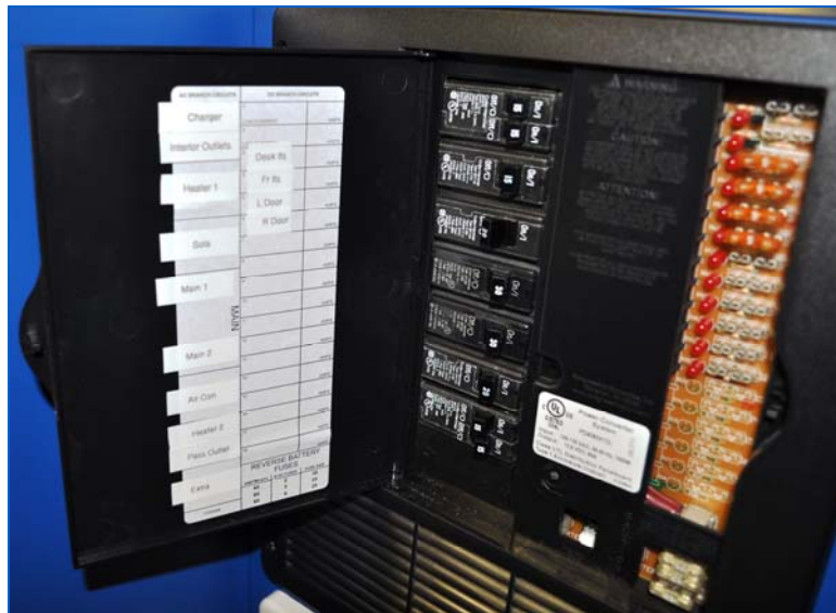
Figure 41: Circuit Breaker Panel and Power converter inside Cabinet
