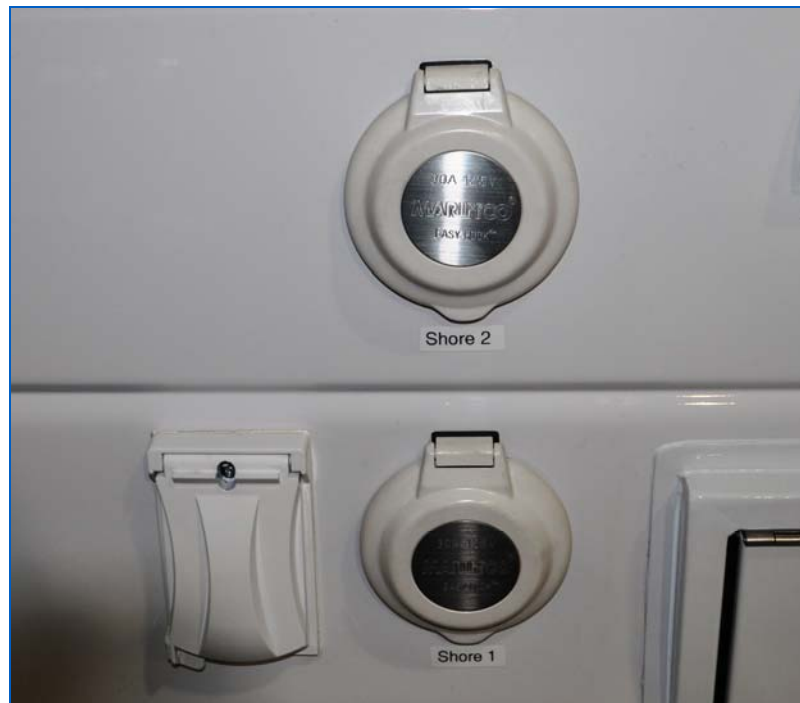
Figure 18: Power Outlet and Shore Power (#1 and #2)
