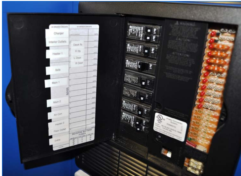
Figure 325: The Power Control Center (Circuit Breaker Box)
