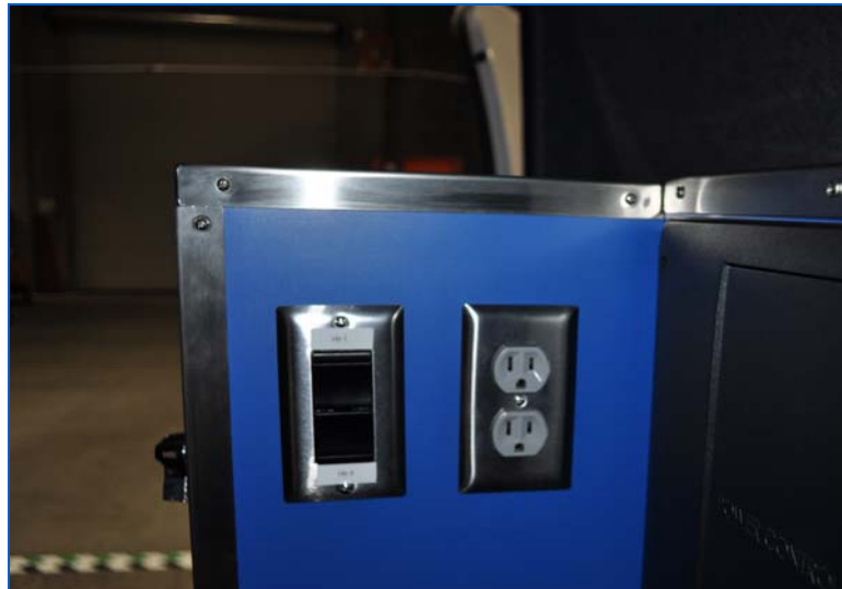
Figure 39: Heater Control and Electrical Outlet
