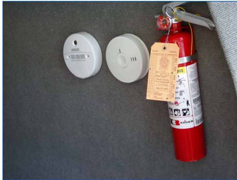
Figure 49: Fire Extinguisher, Carbon Monoxide and Smoke Alarms
