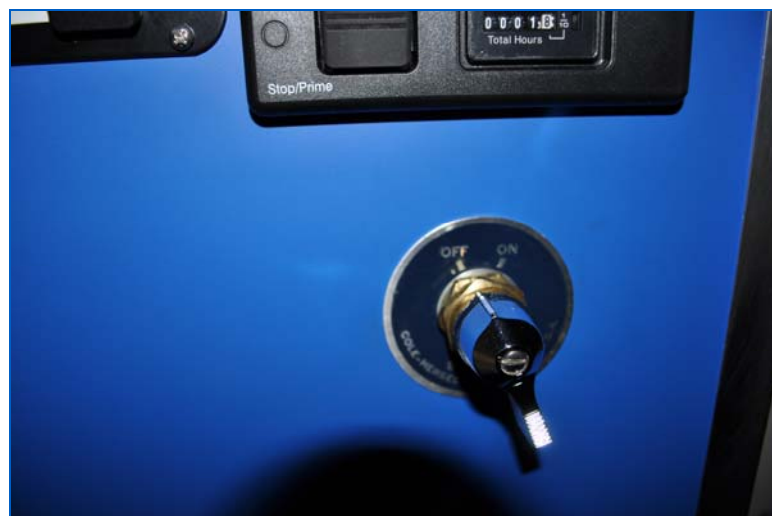
Figure 74: Master Battery Disconnect
