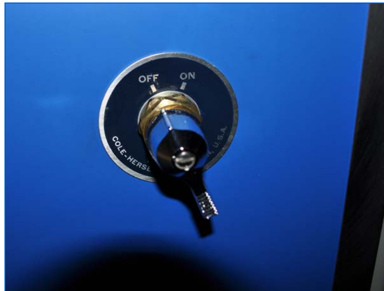
Figure 38: Master Battery Disconnect
