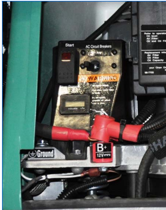
Figure 20: Local Generator Controls
