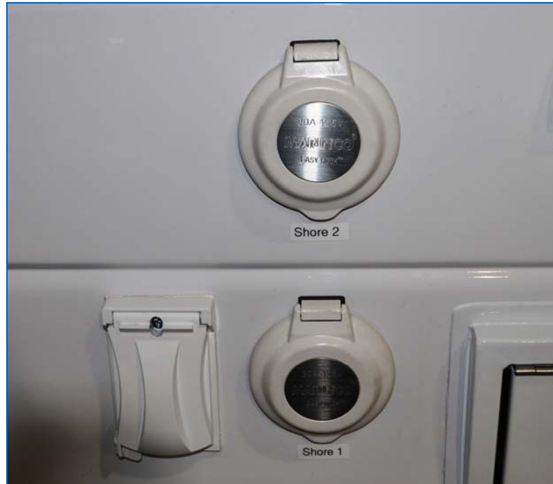
Figure 18: Power Outlet and Shore Power (#1 and #2)
