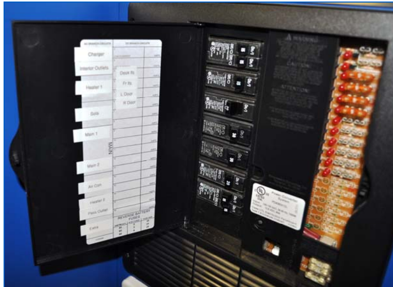
Figure 41: Circuit Breaker Panel
