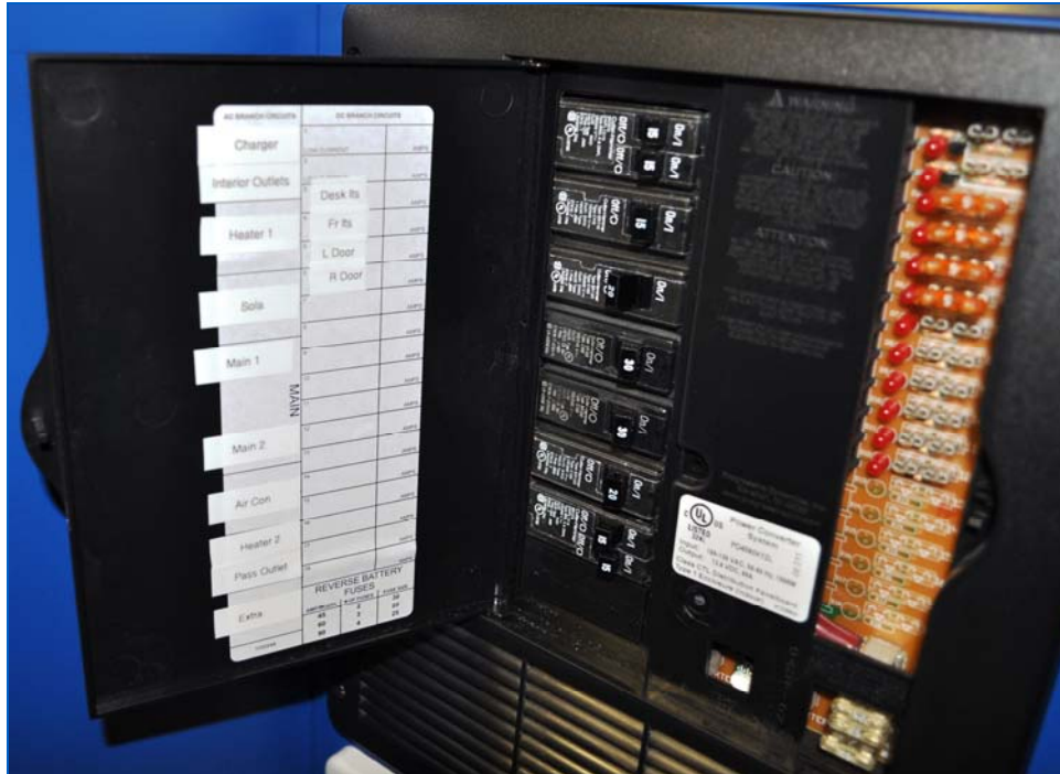
Figure 356: The Power Control Center (Circuit Breaker Box)
