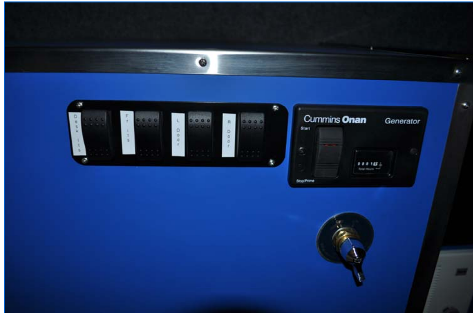
Figure 35: Light Switches, Remote Generator Control and Master Battery Disconnect
