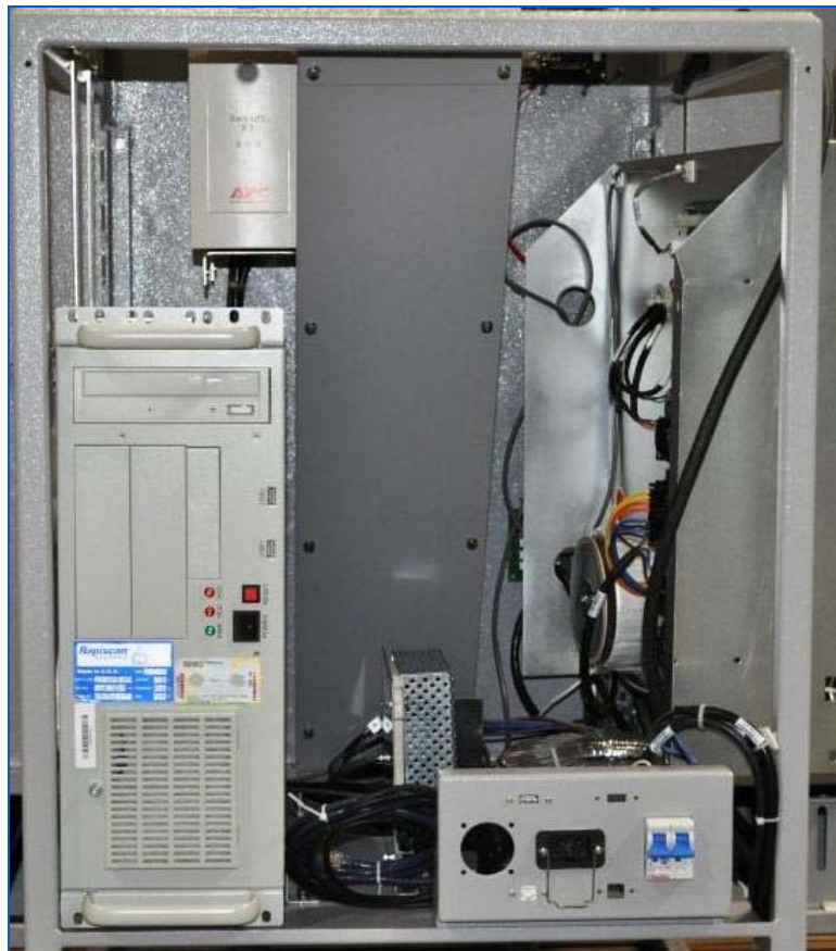
Figure 44: Electronics Cabinet and main circuit breaker
