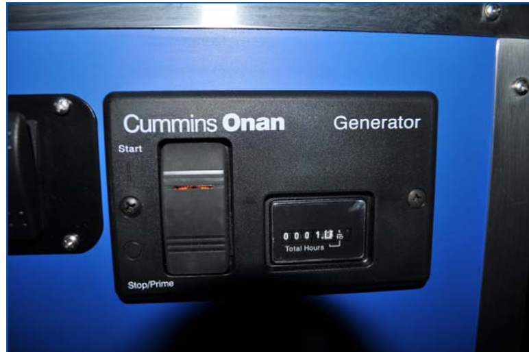
Figure 73: Remote Generator Start-up
