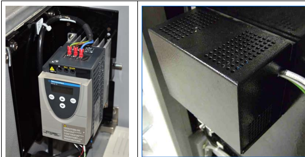
Figure 340: Telemecanique Inverter and Cover
