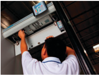
Ready to service and support all field installations
